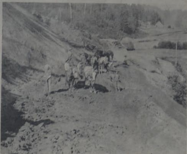
SHOWN ABOVE are construction workers in the process of building Dutch Canyon Road around 1900. Note that teams of horses and mules were used to move the dirt and the only tools available to the hard working men were pick and shovel, not the easiest way to build a road!
