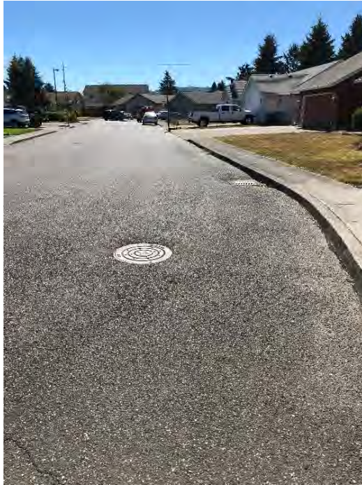
Site location: 8 Photo number: IMG_0711 Description: Inlet and manhole/drywell that is failing, looking south.
