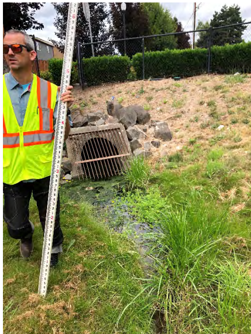
Model ID: INF10_D06_INF10_D04 (Dutch Canyon Infiltration Facility) Photo number: IMG_7882 Description: Standing water present in facility near inlet structure
