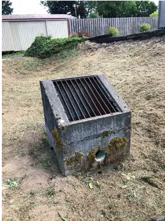
Facility Name Goss Subdivision Photo number: IMG_7916 Description: Outlet structure, two orifices shown
