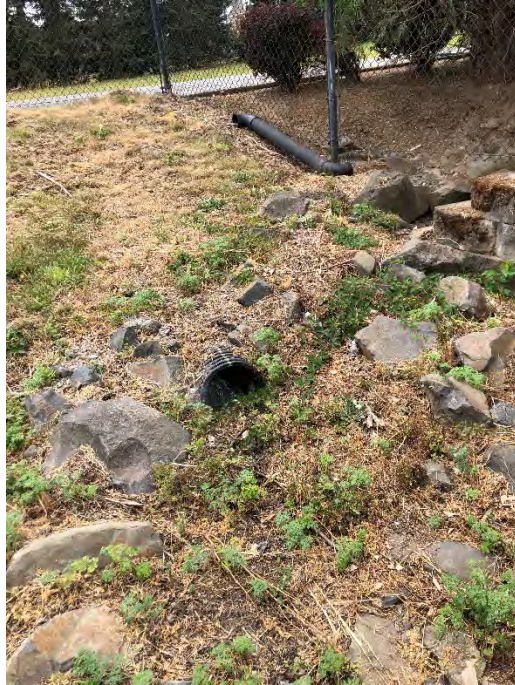
Model ID: INF10_D06_INF10_D04 (Dutch Canyon Infiltration Facility) Photo number: IMG_7886 Description: Lateral inlet from catch basin on corner of Callahan and Old Portland that was observed flooding during Feb 2019 event
