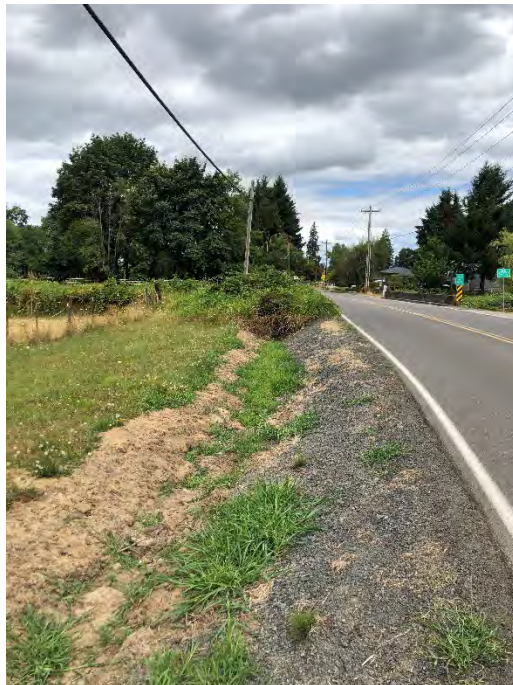
Model ID: SD0591 Photo number: IMG_7899 Description: Most downstream ditch to outfall, which is covered by overgrown bushes.
