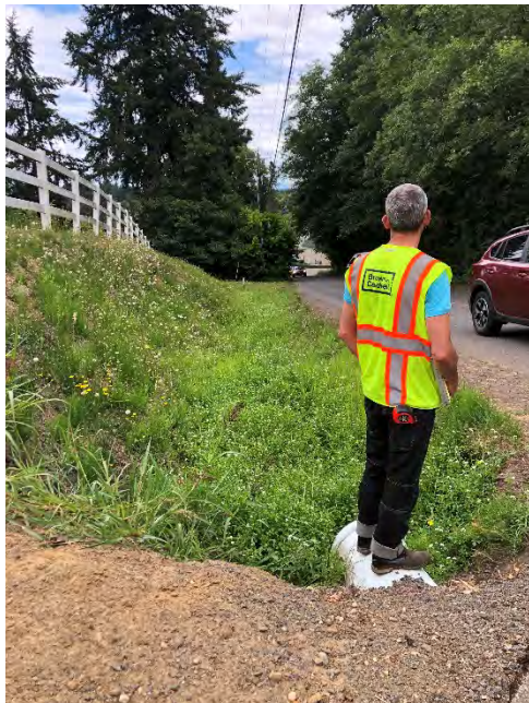
Model ID: SD0742 outfall into SD0740 Photo number: IMG_7905 Description: Culvert into ditch on north side of Keys Road
