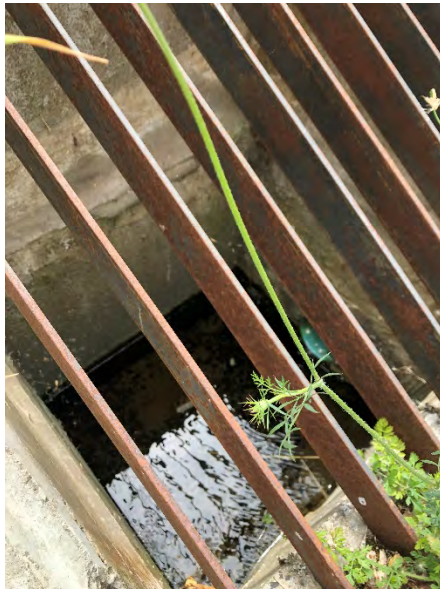
Model ID: South of junction INF10_MH39 Photo number: IMG_7891 Description: Looking down at inlet structure, drain pipe entering from right side of photo (west)
