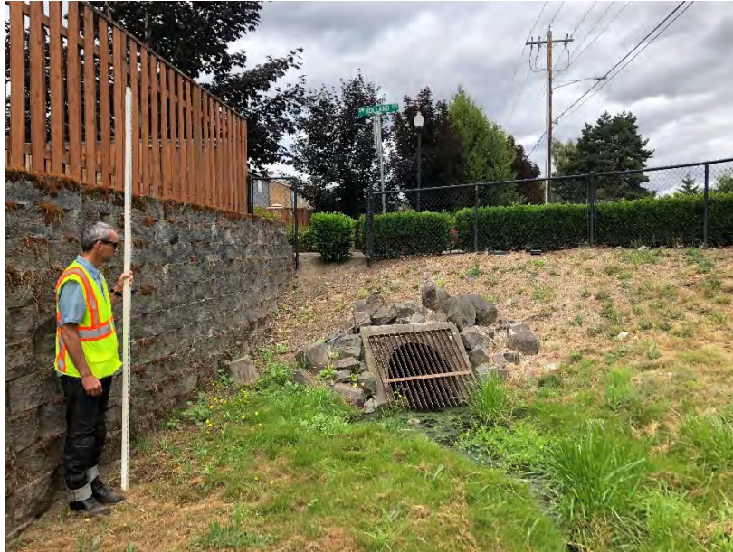
Model ID: INF10_D06_INF10_D04 (Dutch Canyon Infiltration Facility) Photo number: IMG_7880 Description: Looking north at inlet structure, west wall
