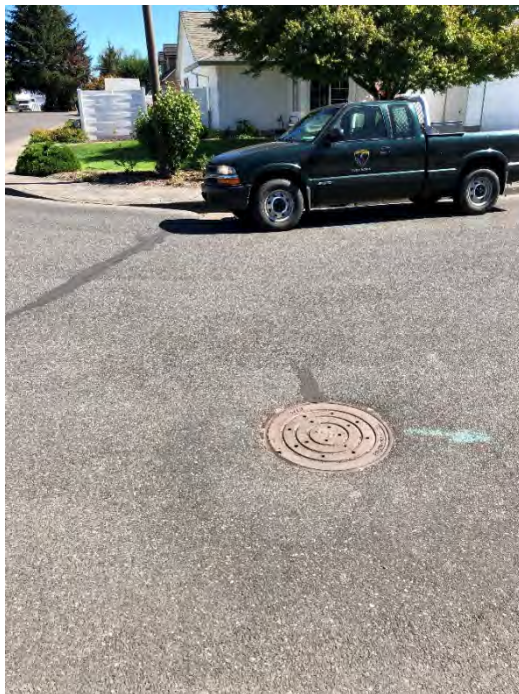
Site location: 8 Photo number: IMG_0712 Description: Inlet (near front tire of truck) and failing drywell, looking east.
