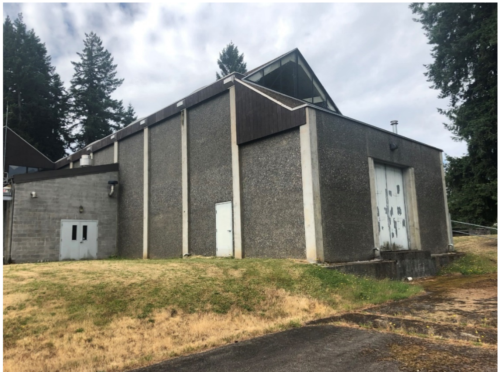
Photo 5: Exposed aggregate precast concrete panels and columns anchorage is nominal and unable to withstand seismic shaking without significant damage at Keys Road.
