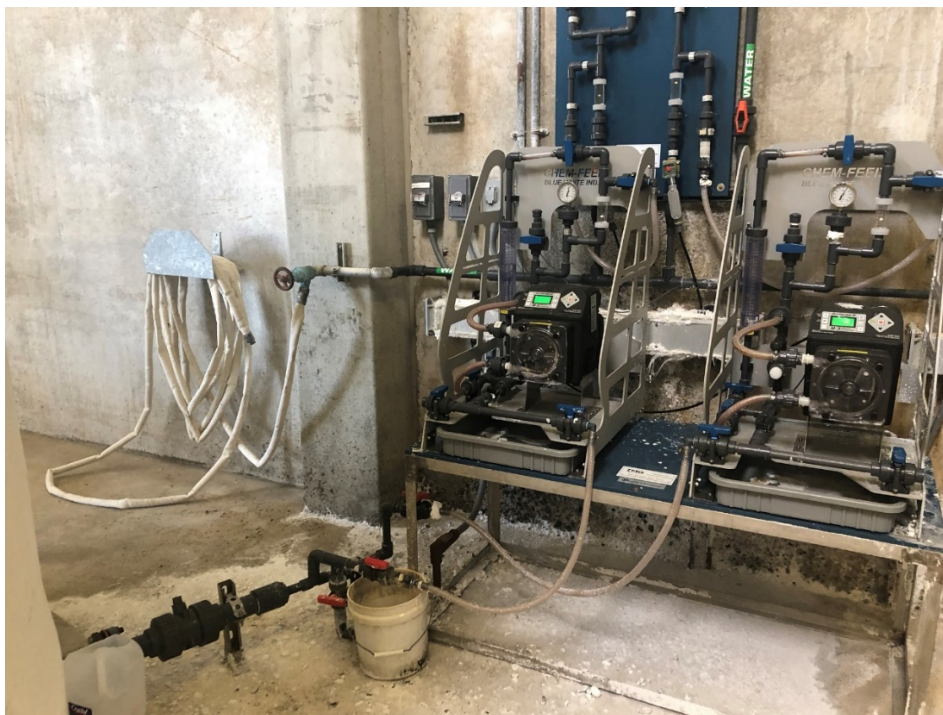
Photo 9: Unanchored chemical metering pumps are likely to experience damage during an earthquake at Keys Road.
