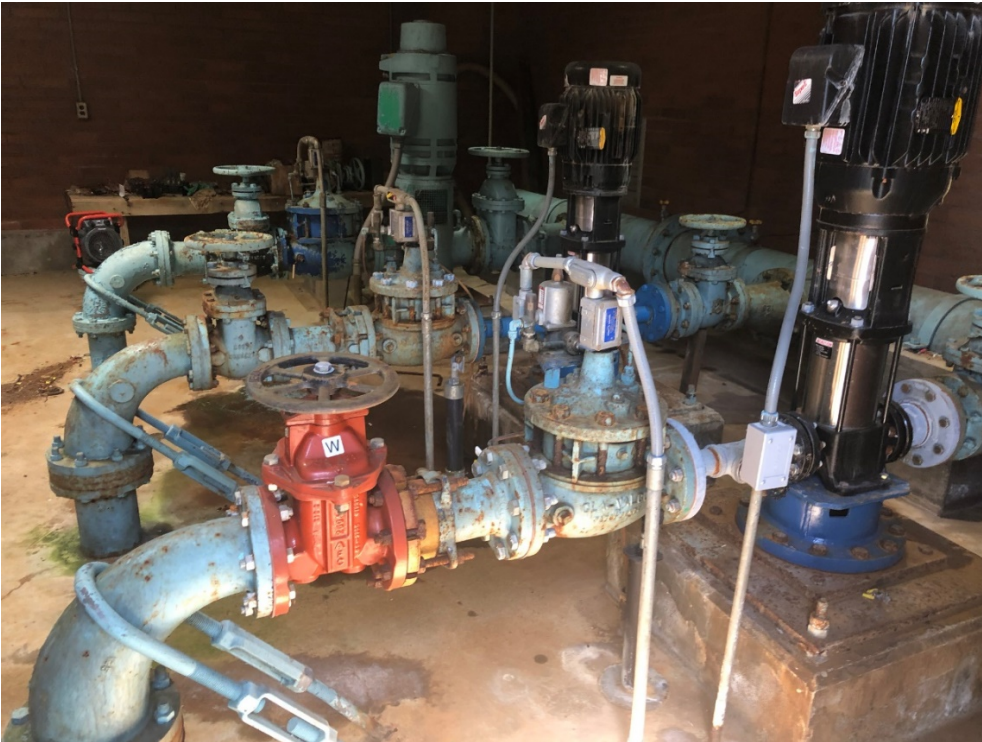
Photo 11: Piping in the Keys Road Pump Station has unusual thrust and lateral restraint systems.
