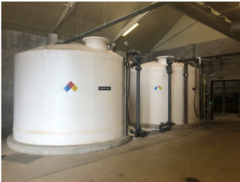
Photo 8: Keys Road Chemical Storage tank anchors are obscured by concrete curb making size and capacity evaluation difficult.
