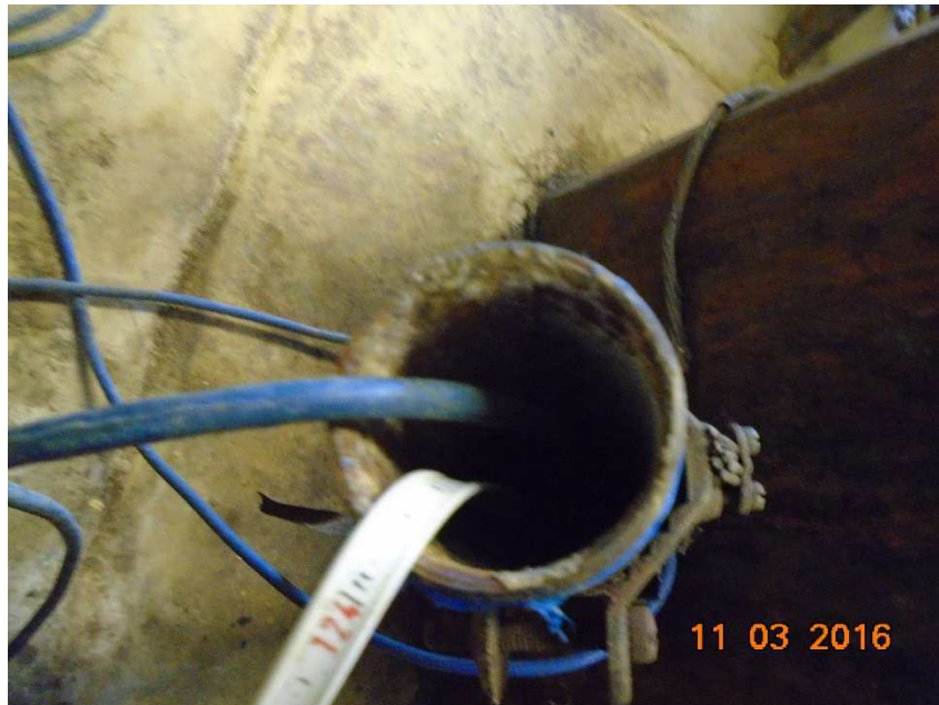
Opening observed in vent in wellhead
