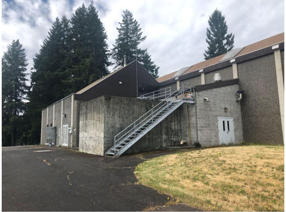
Photo 4: Filter 3 is the exposed masonry block room and cast-in-place tank Treatment Building addition at Keys Road.
