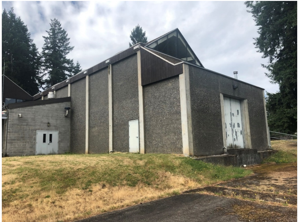
Photo 5: Exposed aggregate precast concrete panels and columns anchorage is nominal and unable to withstand seismic shaking without significant damage at Keys Road.
