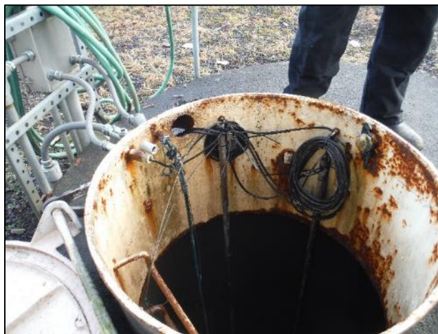
Smith Road Pump Station
