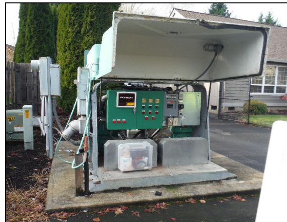
Seven Oaks Pump Station
