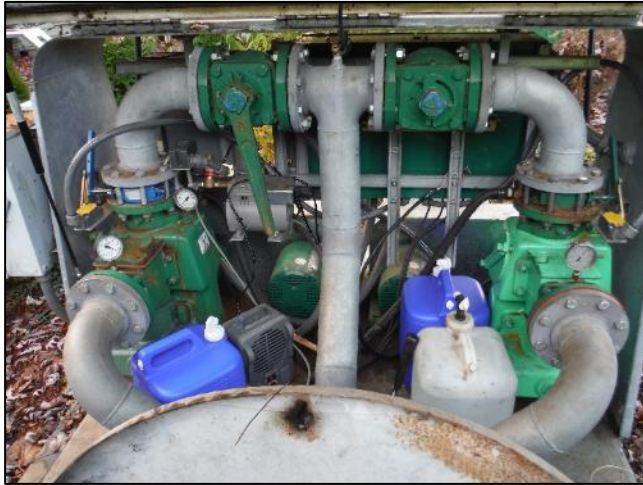
Keys Landing Pump Station
