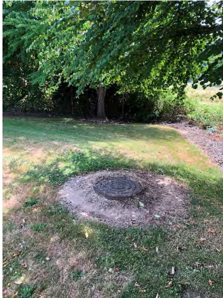
Facility Name Creekview Apartments Photo number: IMG_7910 Description: Manhole after facility outlet, before outfall to Scappoose Creek.
