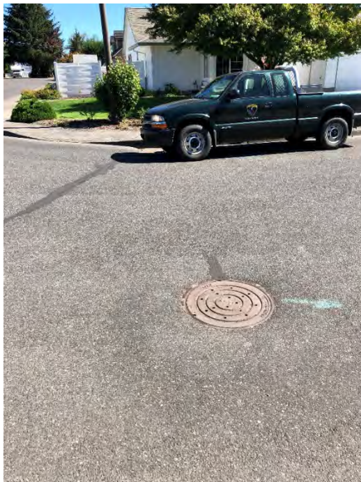
Site location: 8 Photo number: IMG_0712 Description: Inlet (near front tire of truck) and failing drywell, looking east.
