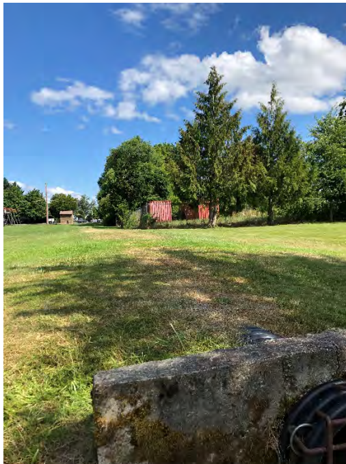
Model ID: SD0724 Photo number: IMG_7926 Description: Mound conveying pipe through Miller Park.
