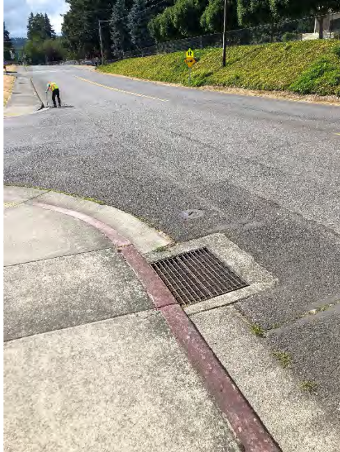
Model ID: DW37_CB02 Photo number: IMG_7933 Description: Catch basin in curb at corner of parking lot, looking west. Pipes visible in basin from east, west, and south.
