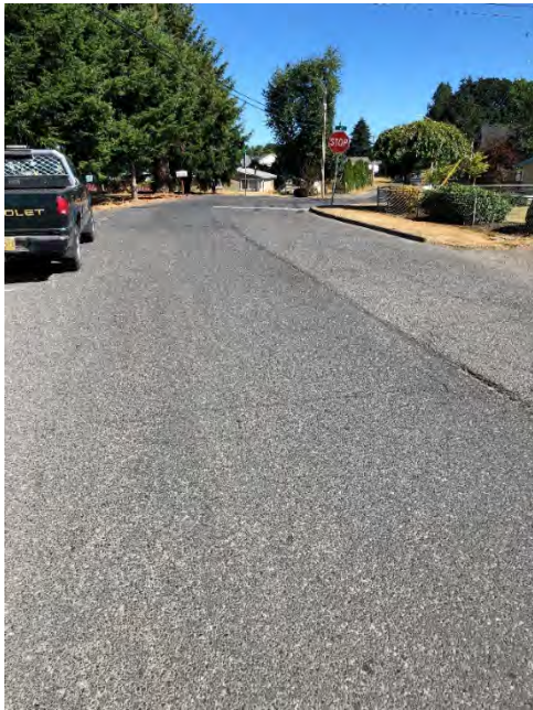
Site Location: 3 Photo number: IMG_0719 Description: Looking west along Elm Street. Driveway on right side floods.
