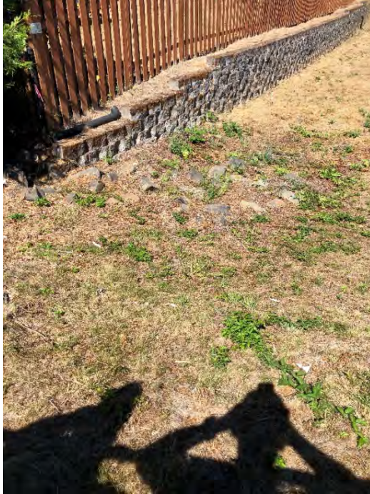
Site location: 28 Photo number: IMG_0689 Description: South end of infiltration facility looking north/northwest
