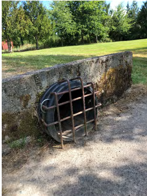
Model ID: PND03_N01 Photo number: IMG_7924 Description: Inlet structure into pipe through Miller Park.
