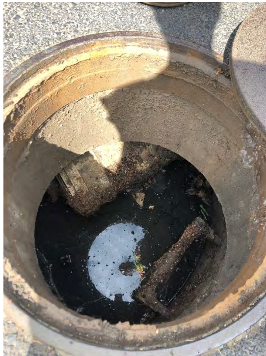
Facility Name Goss Subdivision Photo number: IMG_7918 Description: Water quality manhole upstream of facility, needs cleaning/maintenance
