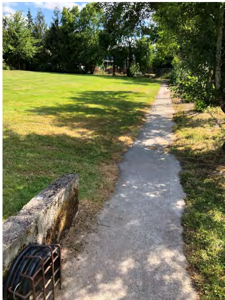
Model ID: PND03_N02_PND03_N01 Photo number: IMG_7925 Description: Drainage pathway that conveys upwelling from CB at sunset loop through to Miller Park. Inlet structure into pipe through Miller Park.
