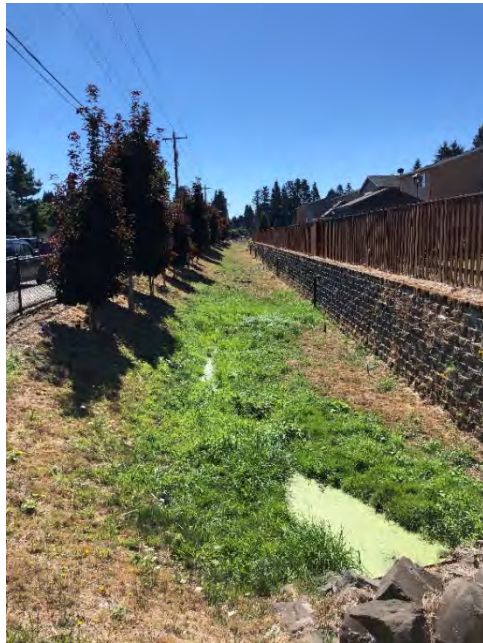
Site location: 28 Photo number: IMG_0686 Description: Large private infiltration facility that receives runoff from multiple neighborhoods and private property as well as roads and public spaces. Looking south.
