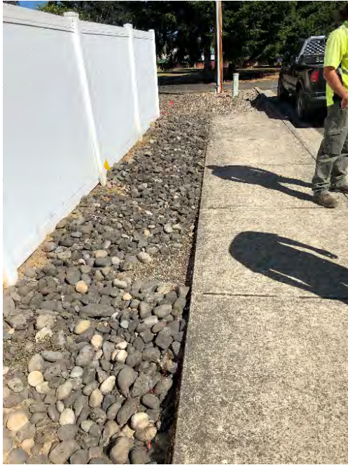
Site Location: 3 Photo number: IMG_0718 Description: French drain looking east along Elm Street.
