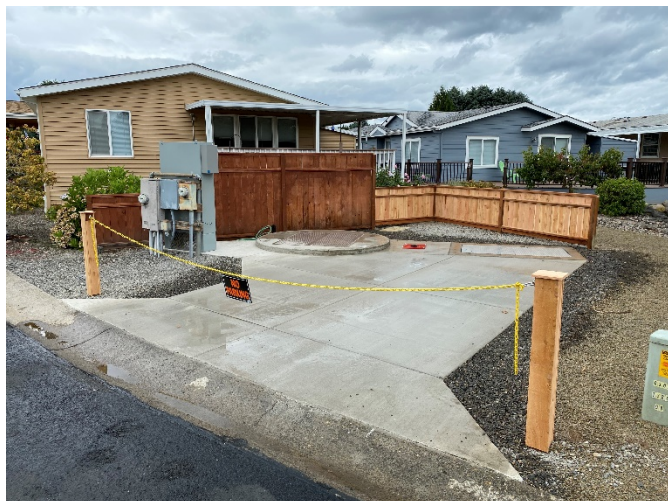
Spring Lake Pump Station
