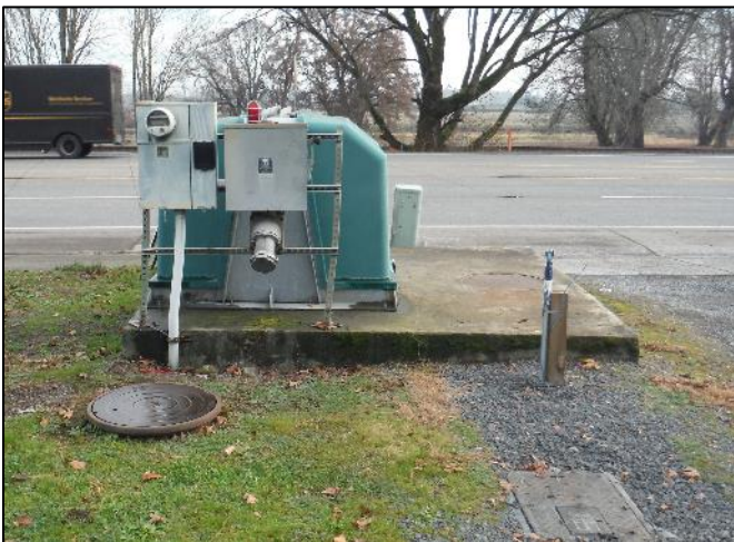
Highway 30 Pump Station
