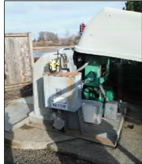
Spring Lake Lift Station
