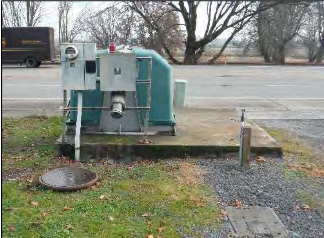
Highway 30 Lift Station
