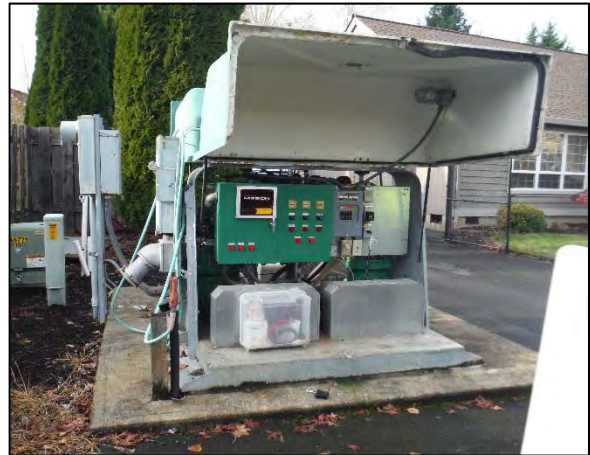
Seven Oaks Lift Station
