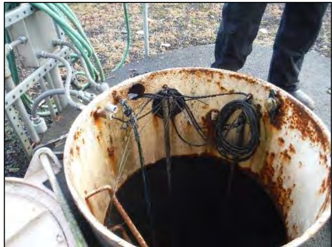
Smith Road Lift Station
