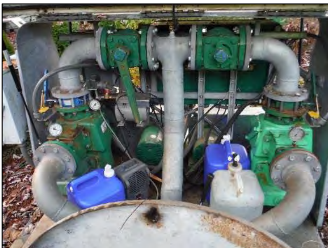
Keys Landing Lift Station
