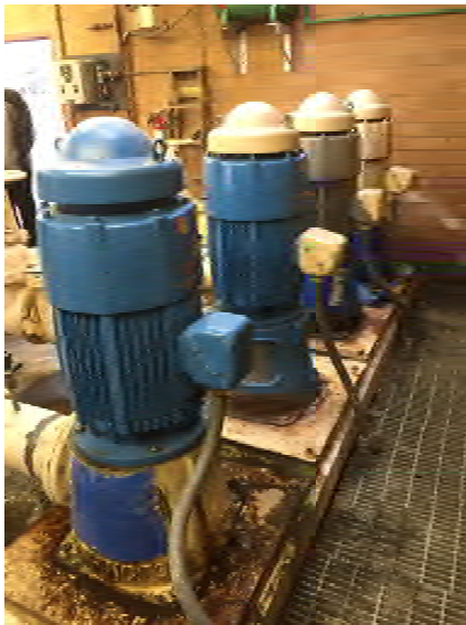
Effluent Pump Station
