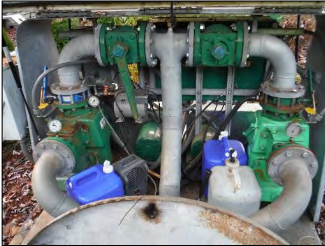
Keys Landing Pump Station
