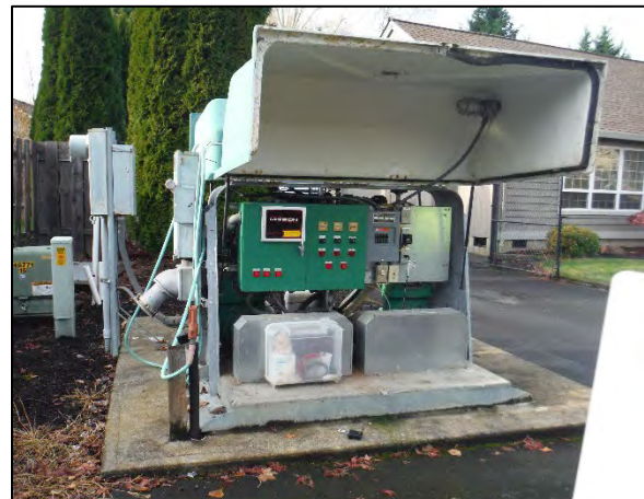
Seven Oaks Pump Station
