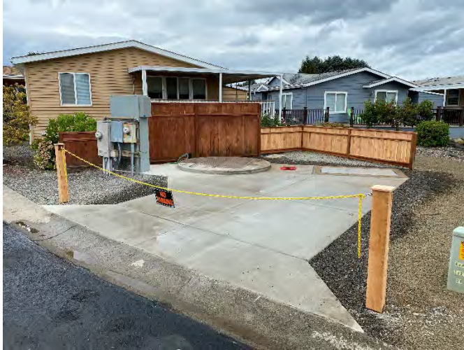
Spring Lake Pump Station
