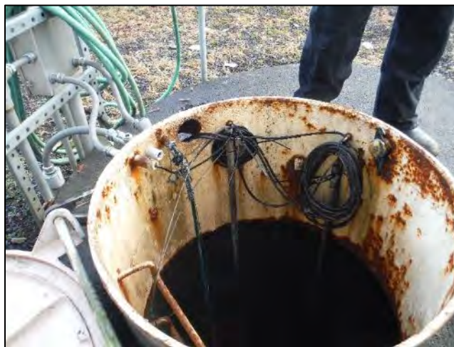
Smith Road Pump Station
