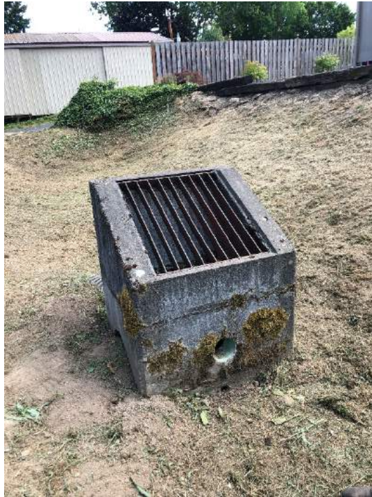
Facility Name Goss Subdivision Photo number: IMG_7916 Description: Outlet structure, two orifices shown
