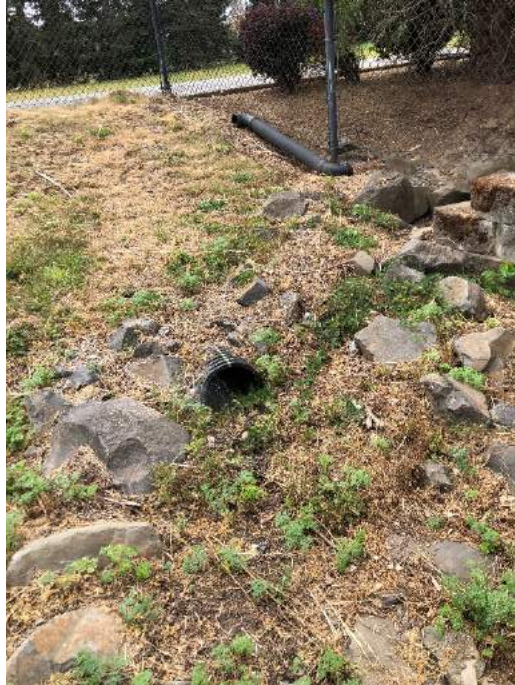
Model ID: INF10_D06_INF10_D04 (Dutch Canyon Infiltration Facility) Photo number: IMG_7886 Description: Lateral inlet from catch basin on corner of Callahan and Old Portland that was observed flooding during Feb 2019 event
