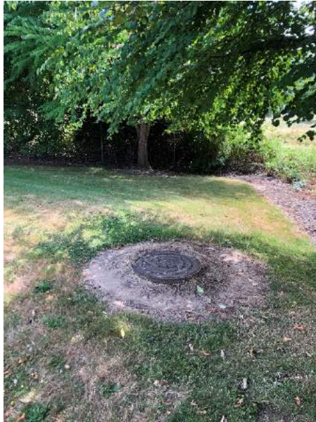
Facility Name Creekview Apartments Photo number: IMG_7910 Description: Manhole after facility outlet, before outfall to Scappoose Creek.
