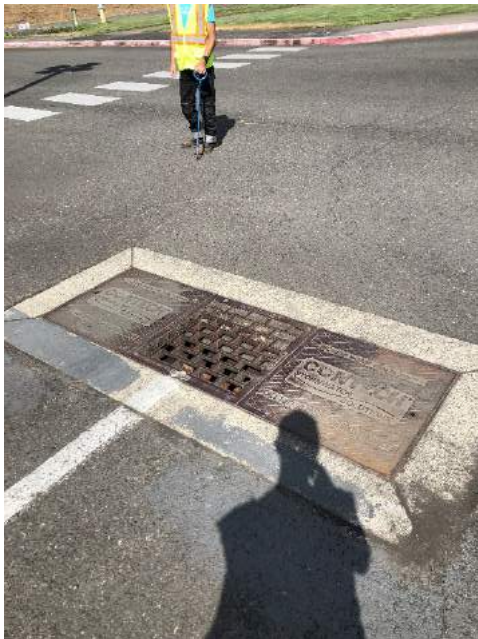
Model ID: N/A Photo number: IMG_7932 Description: CONTECH device in parking lot to south of HS Way.
