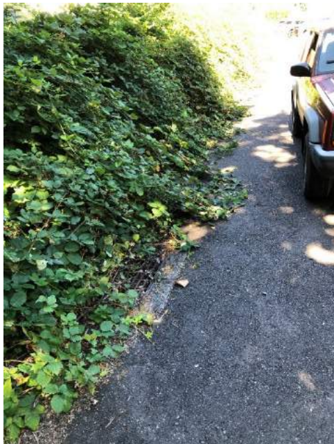
Site location: 10 Photo number: IMG_1784 Description: Inlet covered by vegetation.
