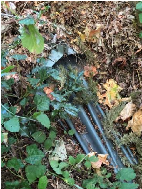
Site location: 16 Photo number: IMG_0681 Description: Storm sock at end of pipe
