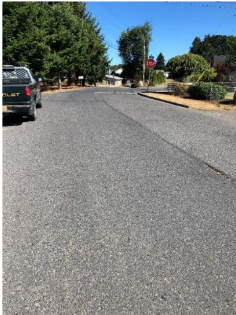
Site Location: 3 Photo number: IMG_0719 Description: Looking west along Elm Street. Driveway on right side floods.
