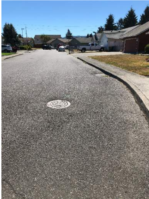
Site location: 8 Photo number: IMG_0711 Description: Inlet and manhole/drywell that is failing, looking south.
