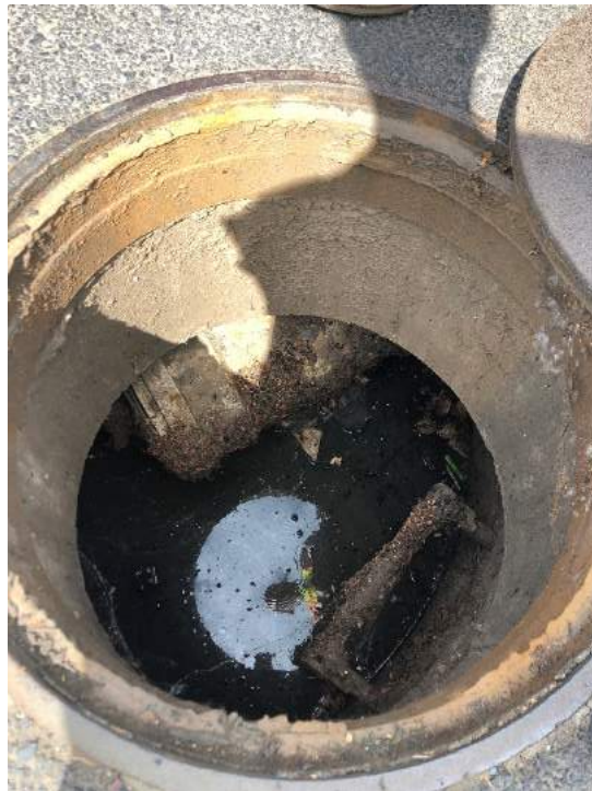
Facility Name Goss Subdivision Photo number: IMG_7918 Description: Water quality manhole upstream of facility, needs cleaning/maintenance
