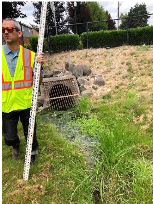
Model ID: INF10_D06_INF10_D04 (Dutch Canyon Infiltration Facility) Photo number: IMG_7882 Description: Standing water present in facility near inlet structure
