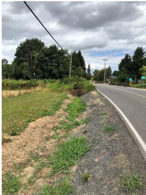
Model ID: SD0591 Photo number: IMG_7899 Description: Most downstream ditch to outfall, which is covered by overgrown bushes.
