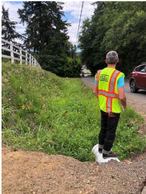
Model ID: SD0742 outfall into SD0740 Photo number: IMG_7905 Description: Culvert into ditch on north side of Keys Road
