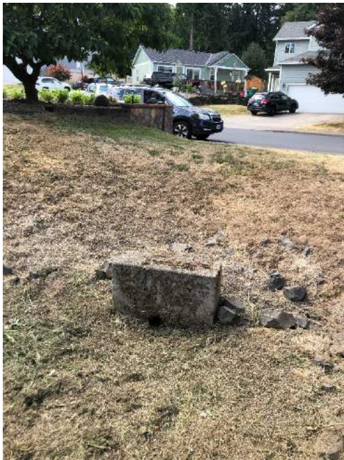
Facility Name Goss Subdivision Photo number: IMG_7914 Description: Inlet structure DS of WQ manhole into facility
